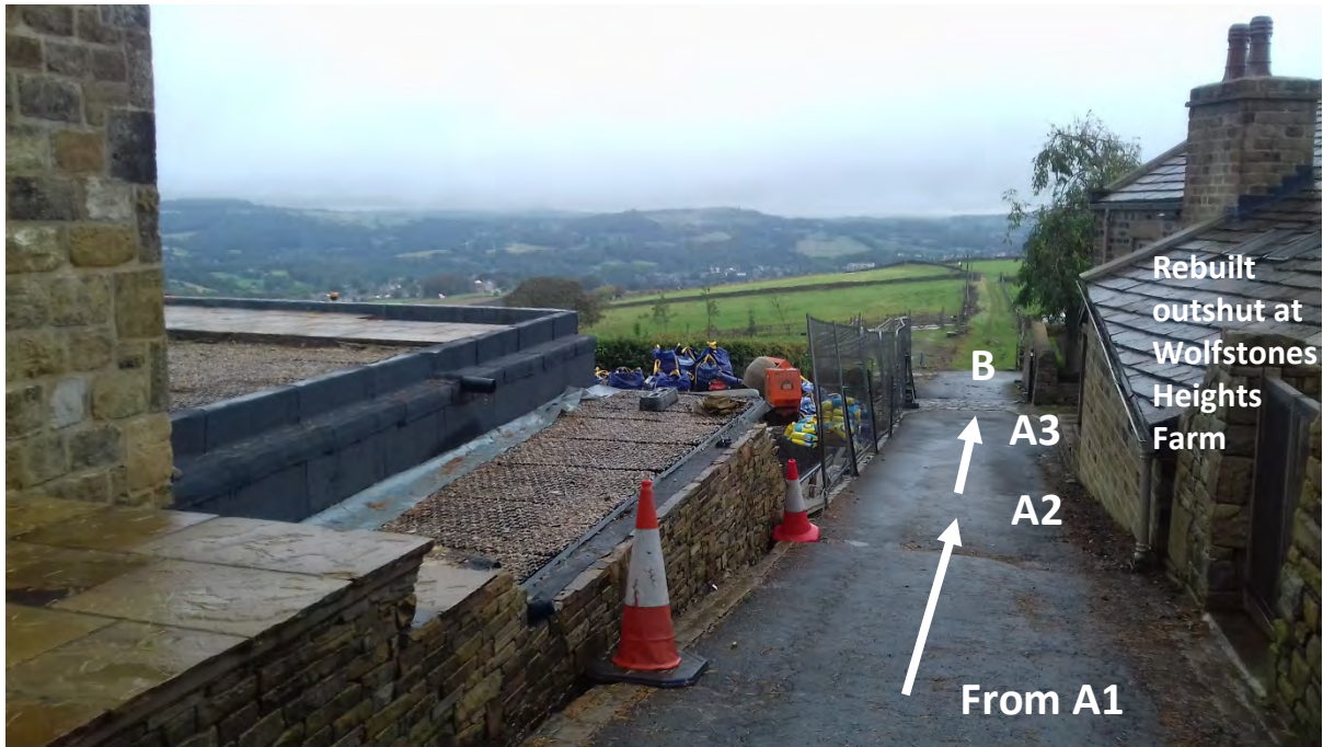
15. View from east to the rebuilt outshut at A2, corner of house at A3 and open gates at B. Work was ongoing to construct garages and related structures to the north of the driveway, however the driveway itself and the continuation to the east were free of building materials or other obstructions etc. 04 Oct 2019.
