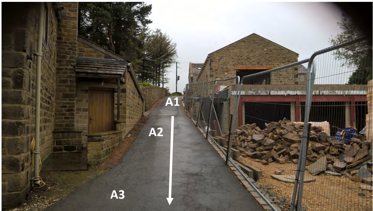
16. View east from the corner of the house at A3, looking west up the driveway toward point A. Similar position to above at A1 looking towards point A. The fire damaged outshut at A2 had been rebuilt. Work was underway to construct a new garage block on the north side of the driveway. 11 Jun 2019.
